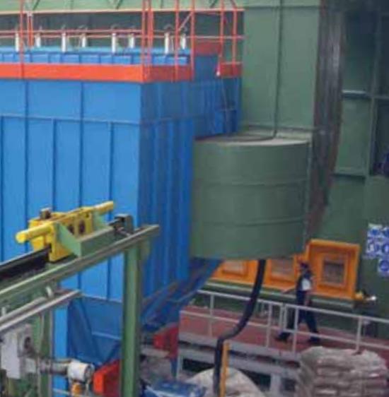
^ Suction and treatment of white fumes from the closed galvanizing bath area.
